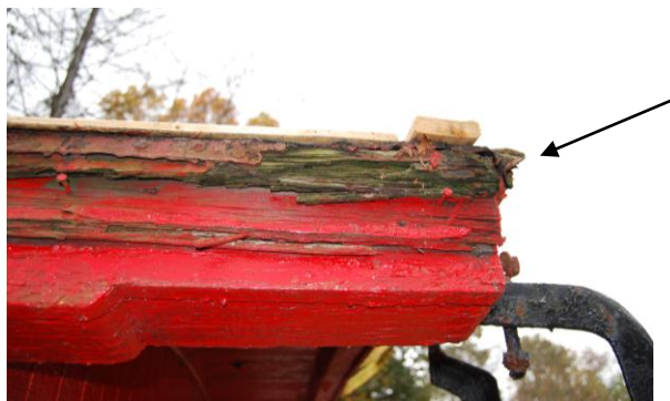
The roof framing is rotting away.
