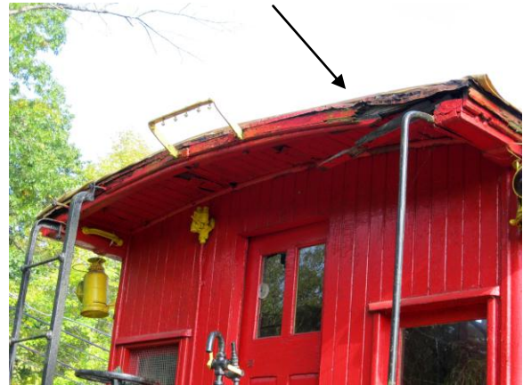
The corner of the fascia board is split and hanging loose.
